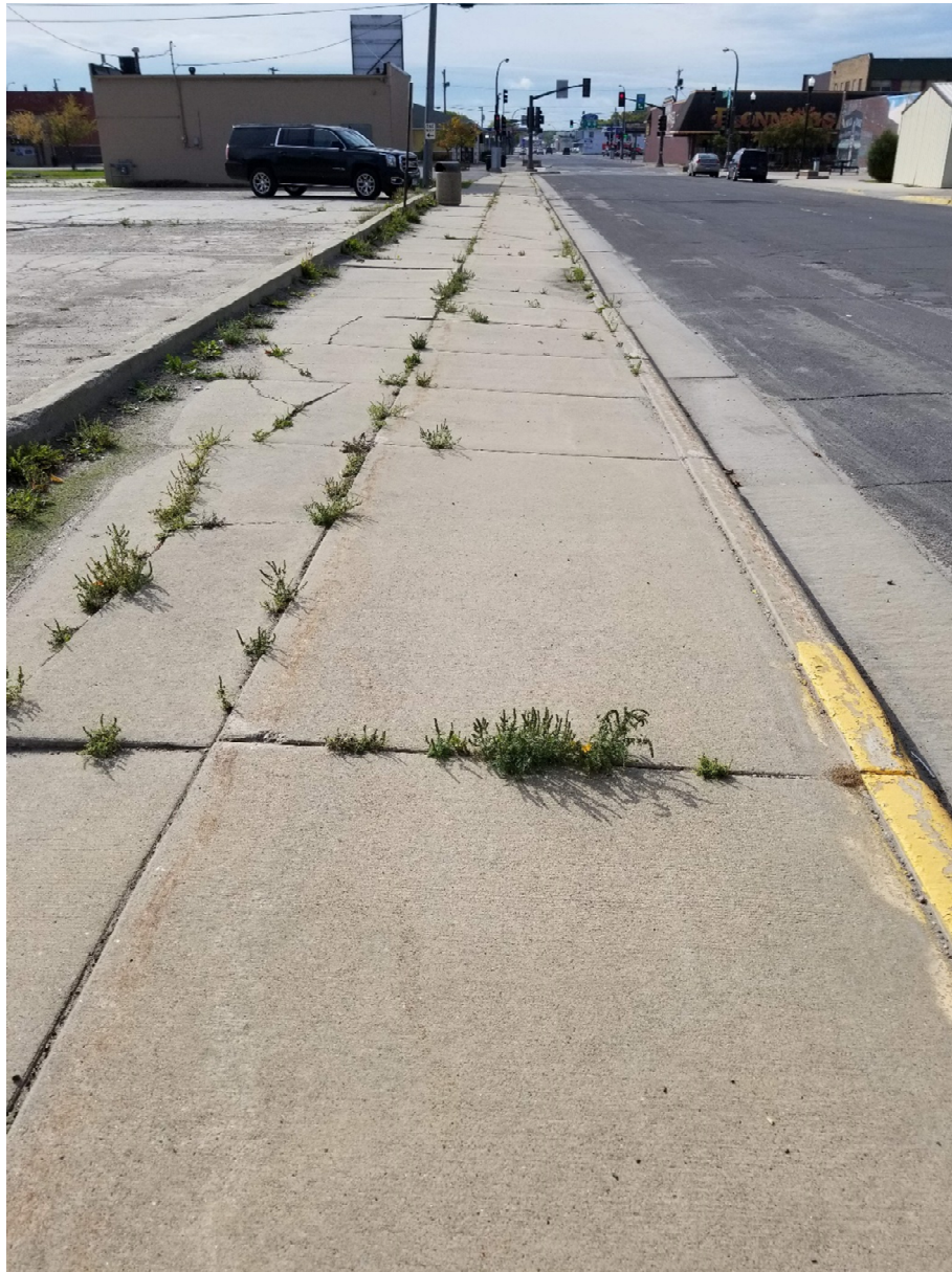
FIGURE 1 NON COMPLIANT SIDEWALK IN INTERNATIONAL FALLS
