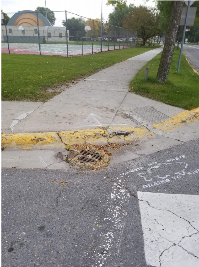
FIGURE 2 NON COMPLIANT CURB RAMP IN INTERNATIONAL FALLS
